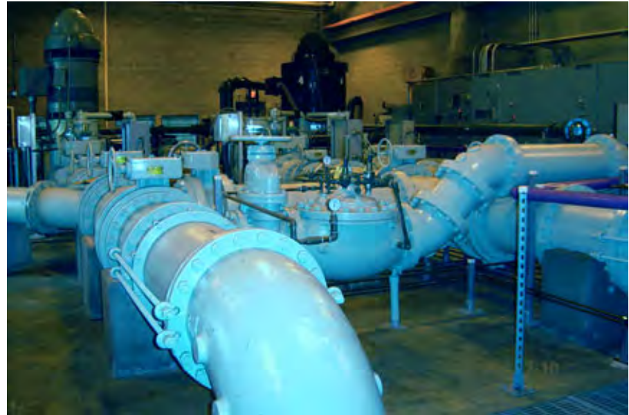
Typical water pumping facility
