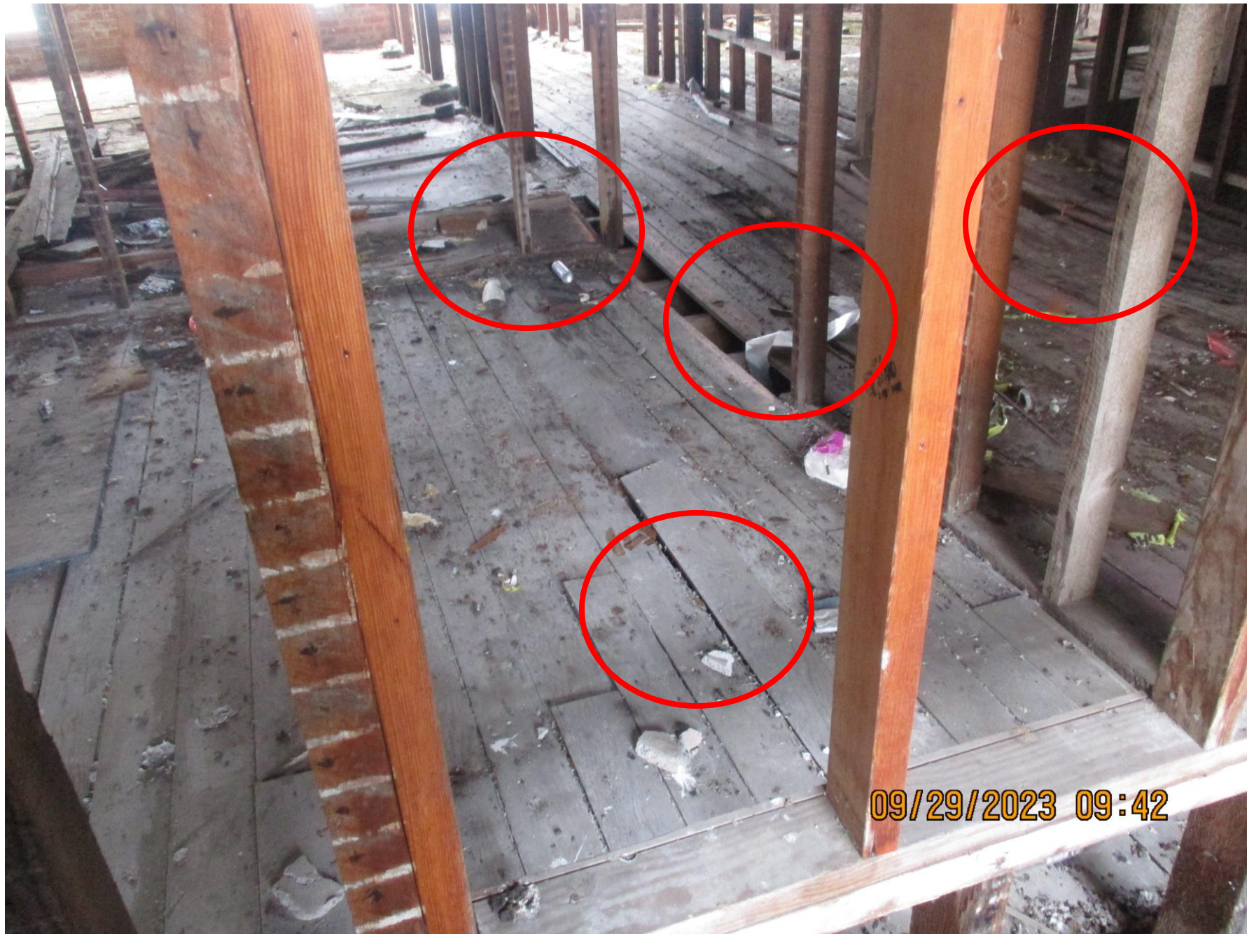
3 RD FLOOR UNEVEN AND COMPROMISED, STATE. DRY-ROT FLOOR ALSO COMPROMISED, STRUCTURAL FAILURE
