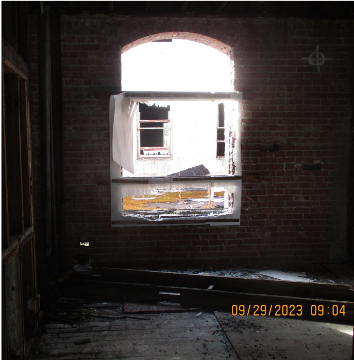
2 ND FLOOR LOOKING AT WEATHER PROOFING FAILURE
