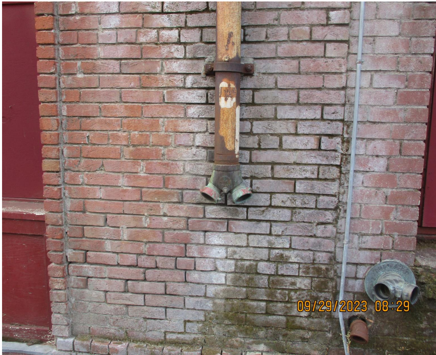
SMITH ST FDC AND STANDPIPE
