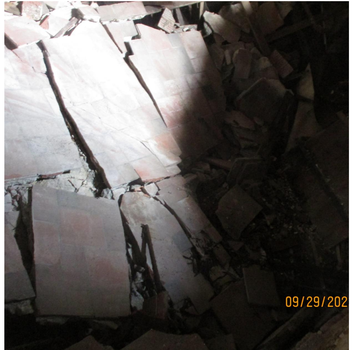
1 ST FLOOR LOOKING AT 1 ST FLOOR, AT STATE ST SIDE OF BUILDING. FLOOR JOIST STRUCTURAL FAILURE
