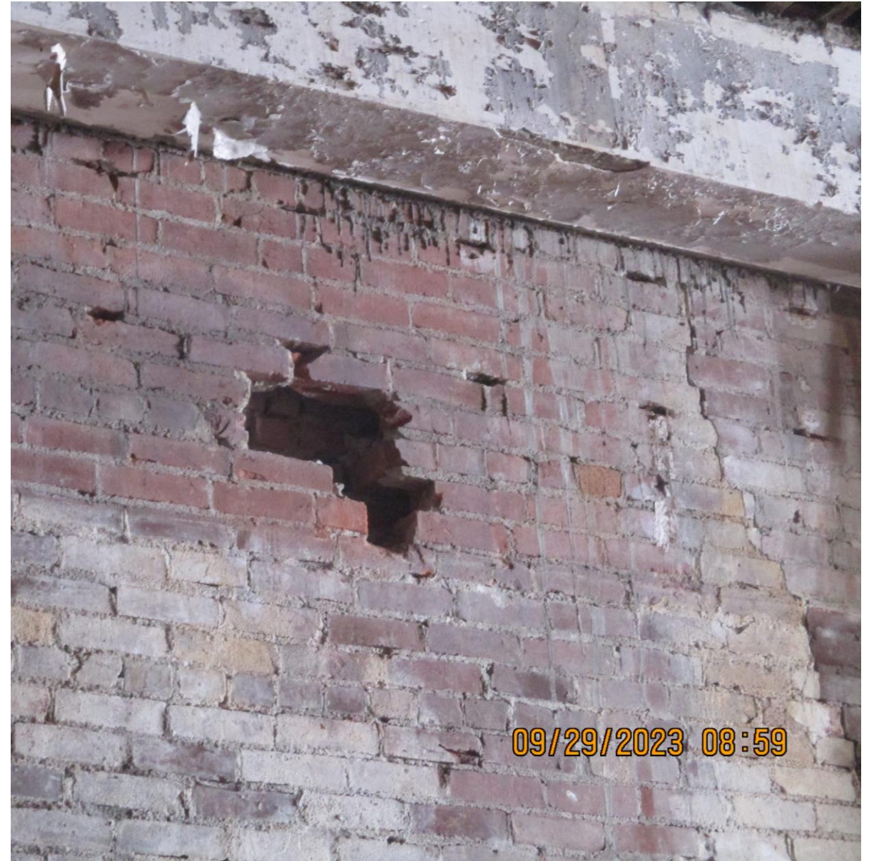
1 ST FLOOR BRICK WALL STRUCTURAL FAILURE
