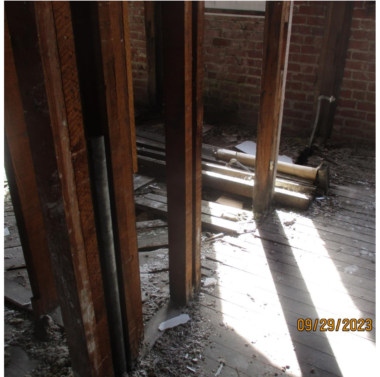
STRUCTURALLY COMPROMISED FLOOR
