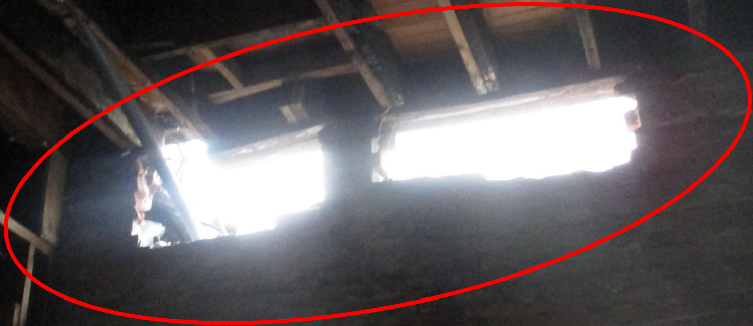
1 ST FLOOR BRICK WALL STRUCTURAL FAILURE
