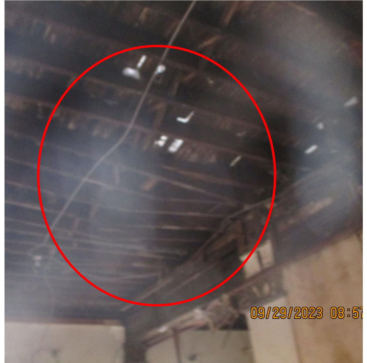
1 ST FLOOR LOOKING AT 2 ND FLOOR, AT STATE ST SIDE OF BUILDING. FLOOR JOIST STRUCTURAL FAILURE
