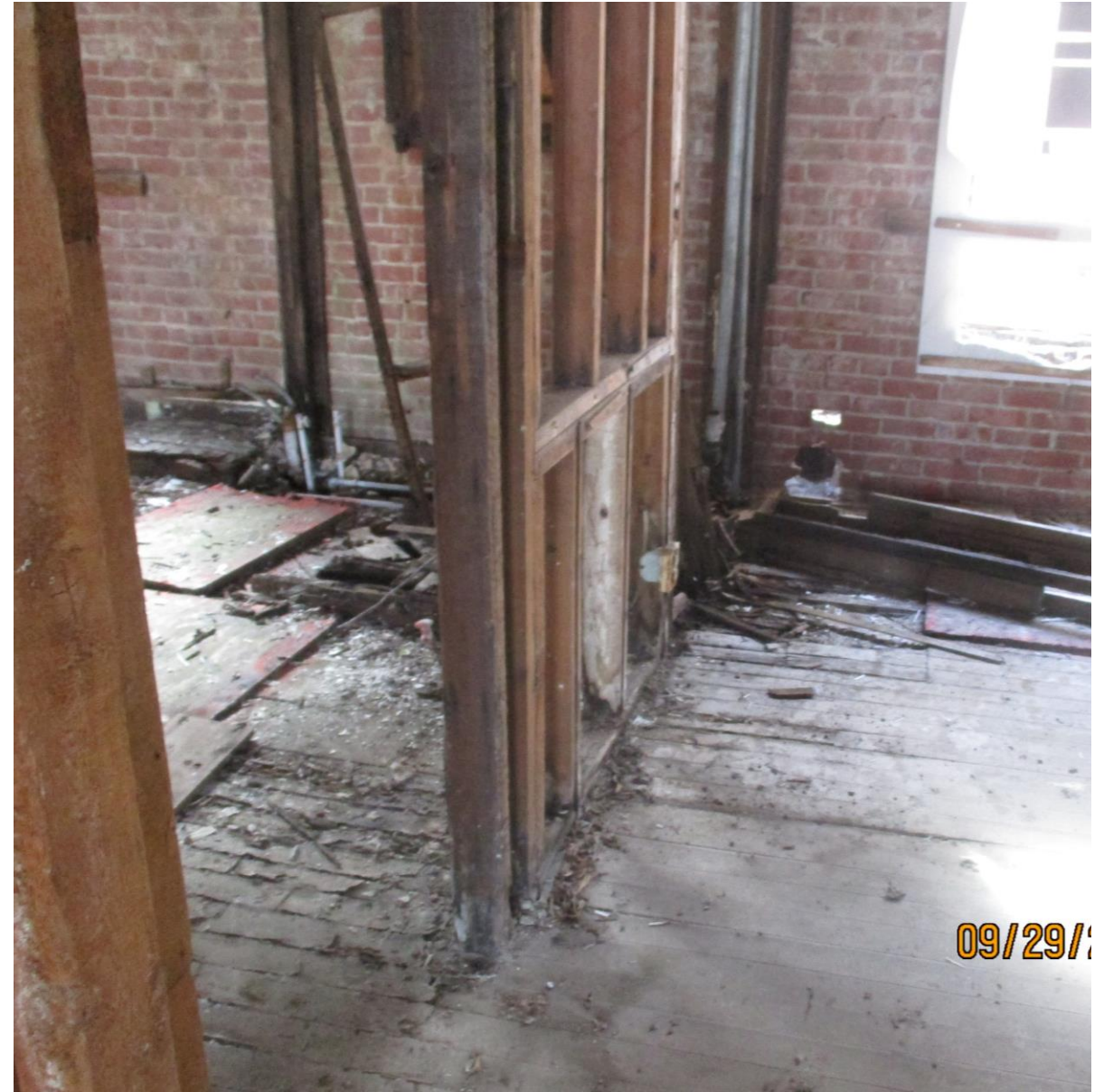
2 ND FLOOR, FLOOR JOIST STRUCTURAL FAILURE, AND ROT
