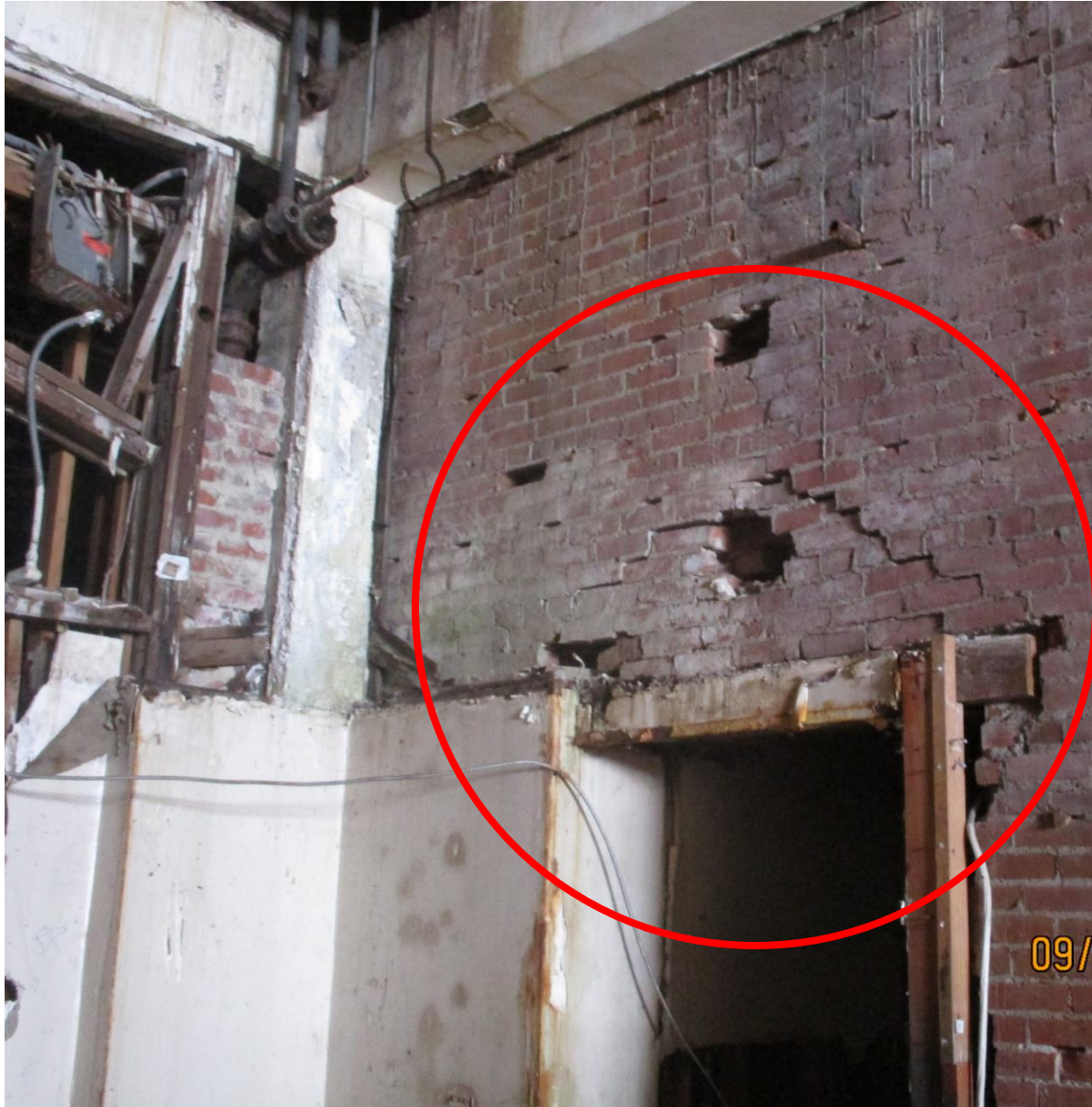
1 ST FLOOR. AT STATE ST SIDE OF BUILDING. BRICK WALL STRUCTURAL FAILURE
