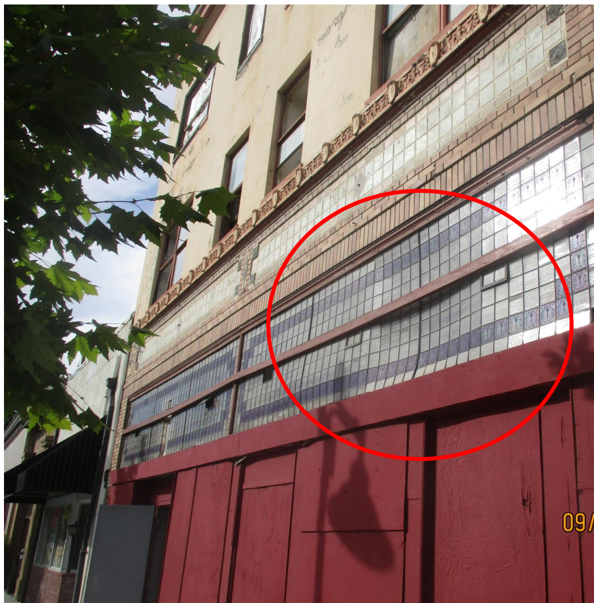
LEAD GLASS FAILURE STATE ST
