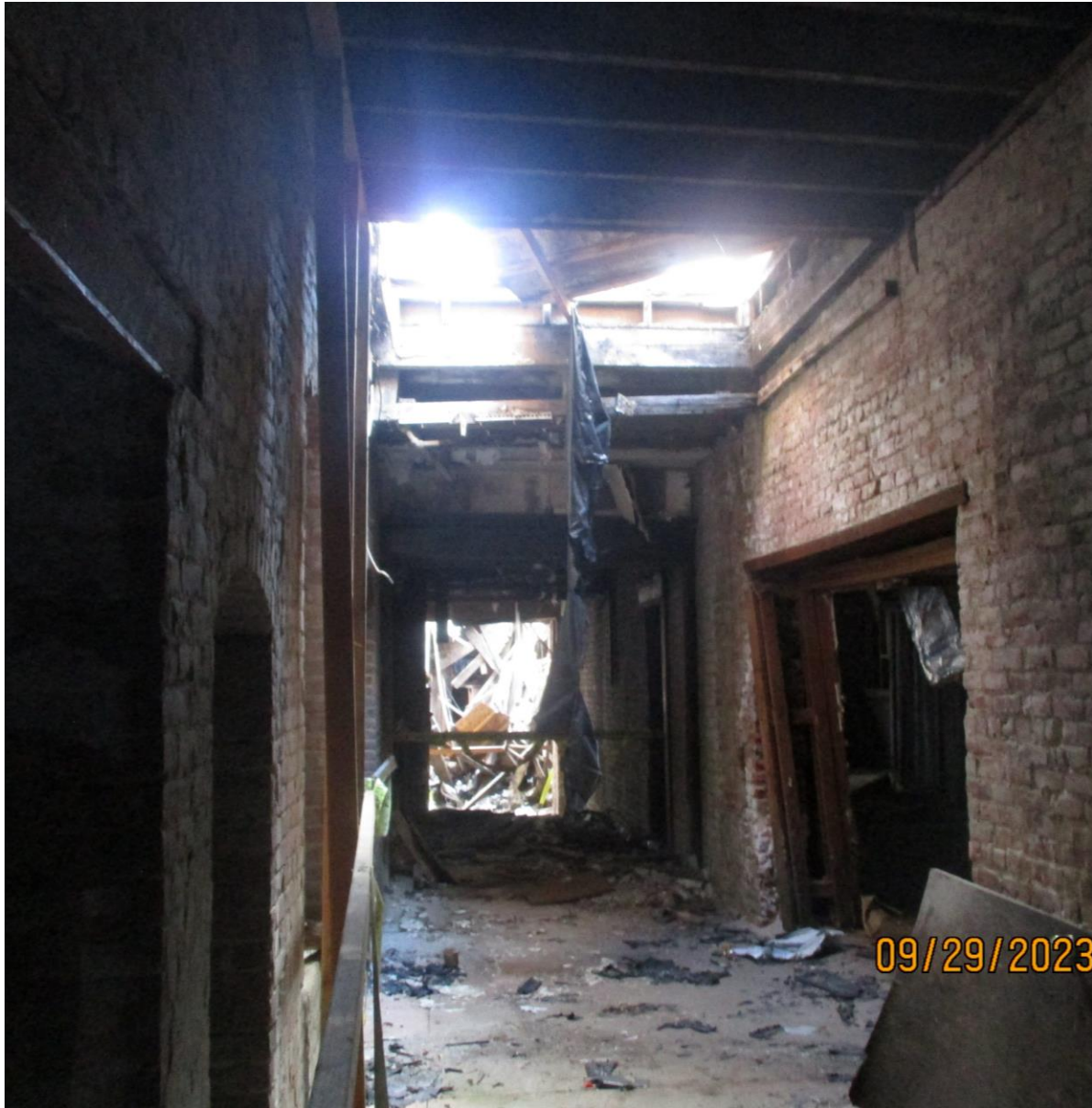
1 ST FLOOR LOOKING THROUGH ATRIUM, FLOOR JOIST STRUCTURAL FAILURE, AND OPEN TO WEATHER.
