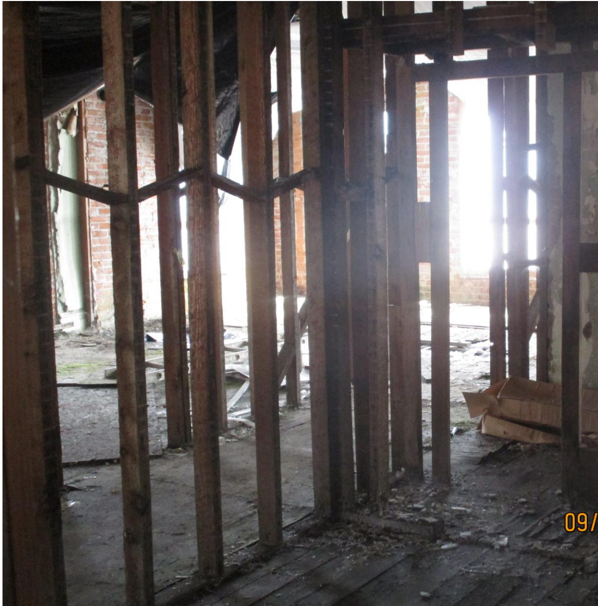
3 RD FLOOR STATE ST SIDE: FLOOR JOIST STRUCTURAL FAILURE, AND ROT
