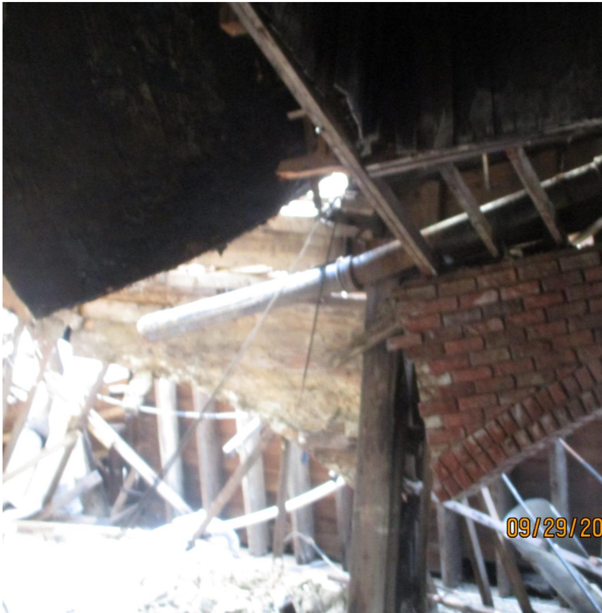
STRUCTURAL FAILURE AND PARTIAL COLLAPSE OF THE ATRIUM ROOF. LOCATION 1 FLOOR.
