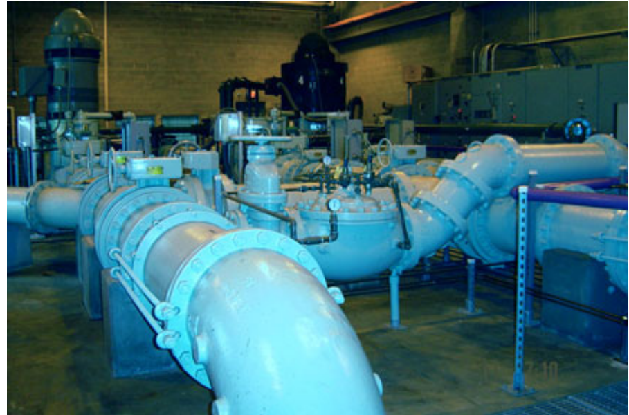
Typical water pumping facility
